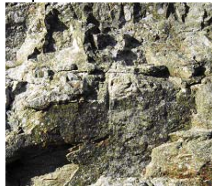
Evidence of boreholes
